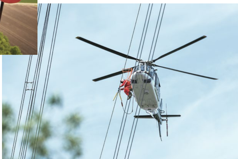
Using a helicopter to help install bird protection measures: the black-and-white markers help the birds better see the conductors.
