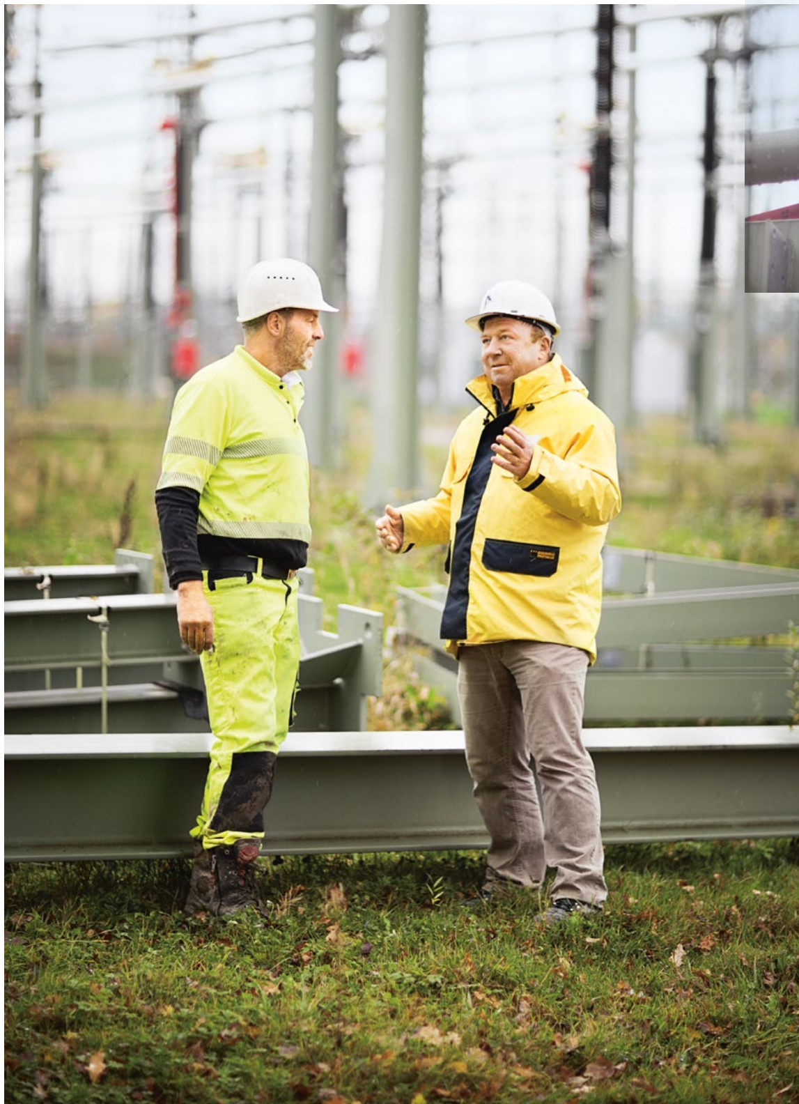
Partners on the construction site: Heckmann site foreman Ferdinand Langenkämper (left) and Amprion site manager Olaf Tietz have been working together in Essen-Eiberg since October 2014.
